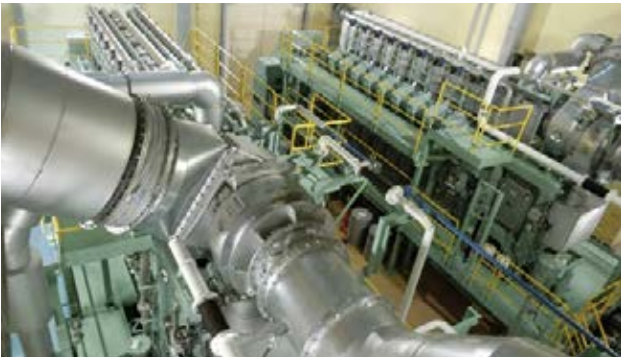
Gas engine power generation facilities
