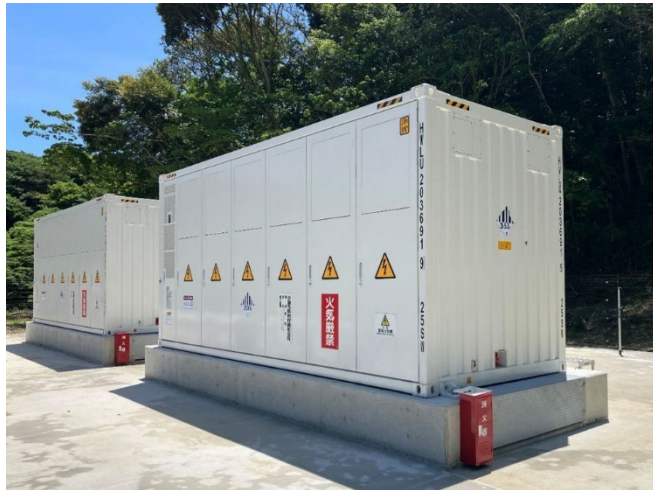
Ichigo Onjuku Iwawada ECO Battery Storage Plant
