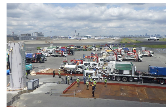
FY2023 ground improvement work for the north side of Runway A and associated taxiways at Tokyo International Airport
