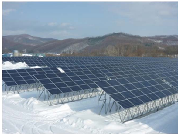
Ichigo Engaru Higashimachi ECO Power Plant (Hokkaido)
