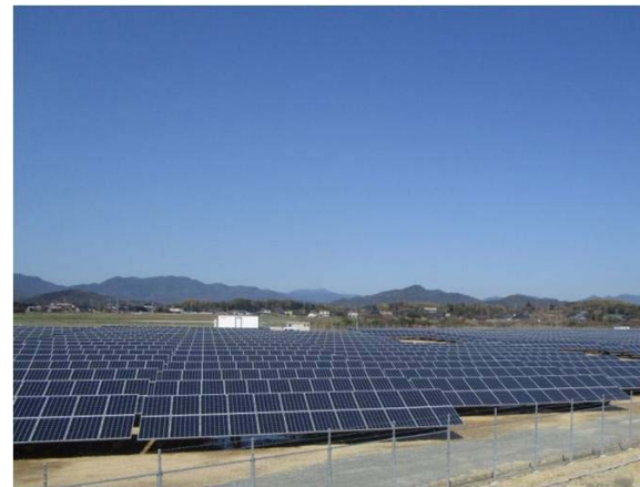
Ichigo Yamaguchi Sayama ECO Power Plant (2.35MW)
